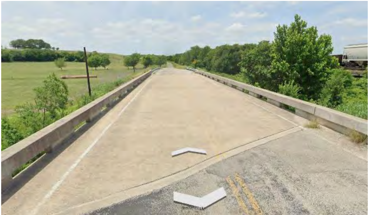
Figure 6 Welch Street would be inundated by about 3.5 feet of floodwaters during a breach of Upper Brushy Creek FRS No. 25
