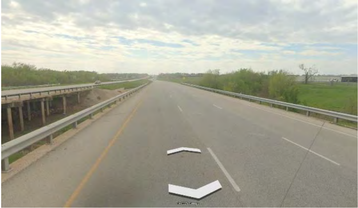
Figure 3 US Highway 79 would be inundated by about 1.5 feet of floodwaters during a breach of Upper Brushy Creek FRS No. 25
